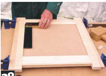
28 Cramp up doors on level surface. Check accuracy with try square or measure across the diagonals
